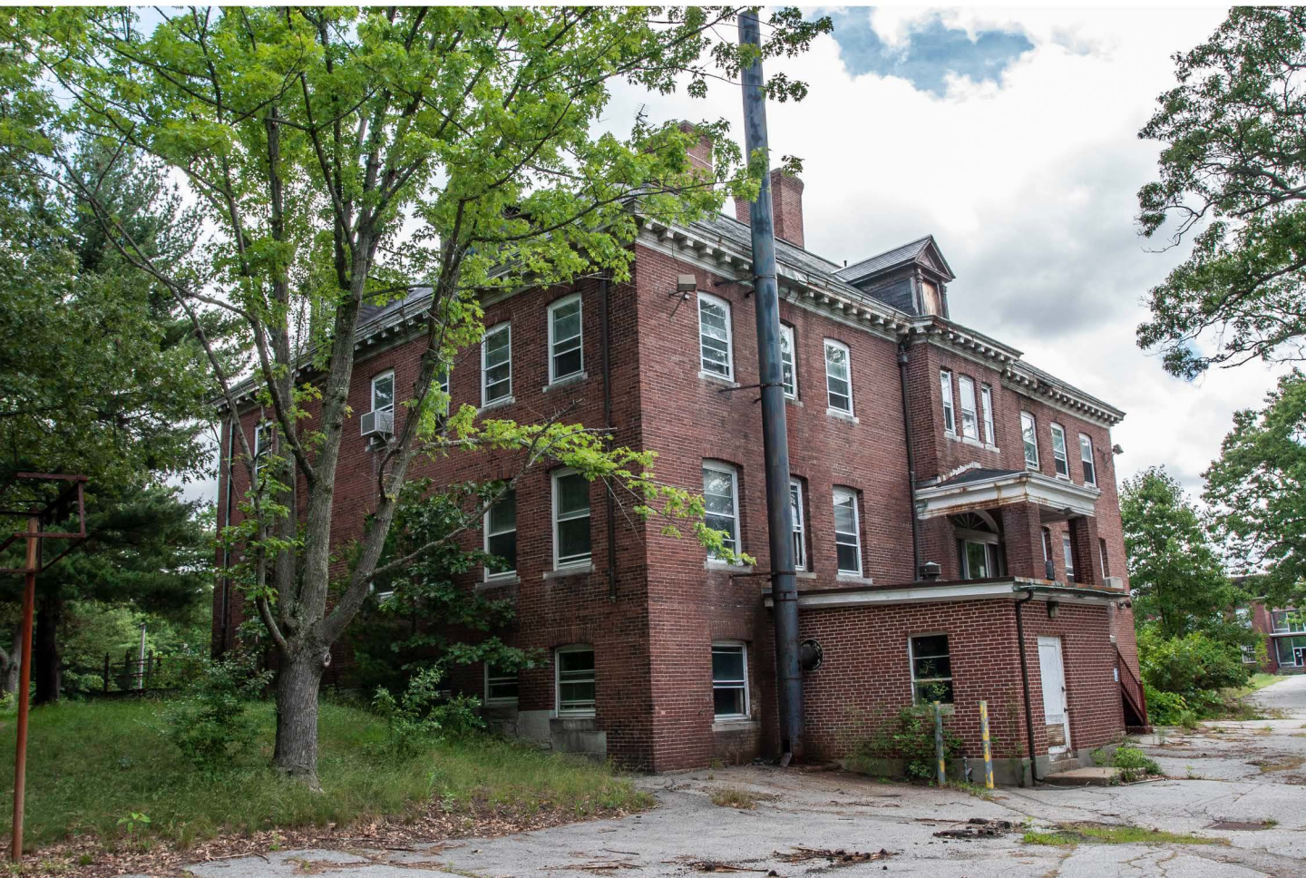
Gould Hall right rear, heating plant stack and boiler room, June 10, 2007
