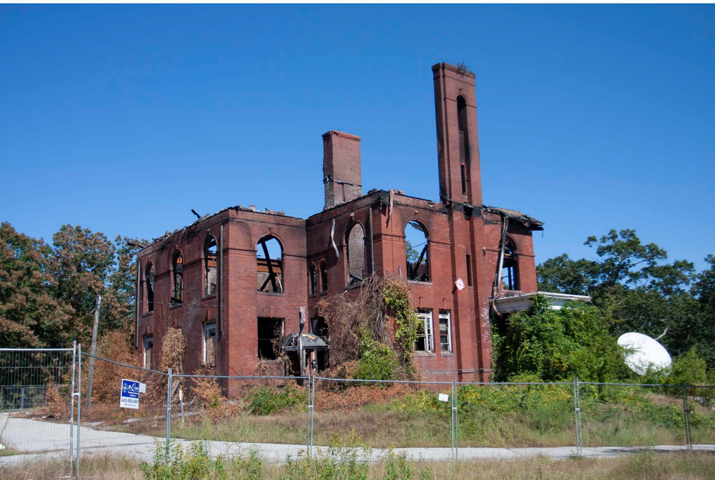
Aftermath of the Read Hall arson fire, September 4, 2013
