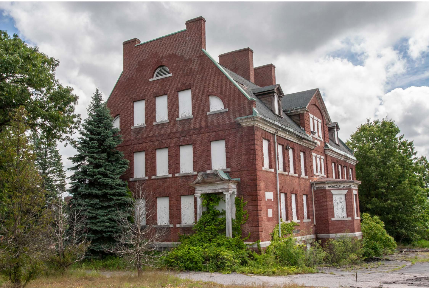
Abandoned Richardson Hall right rear, large holes in roof, June 10, 2007
