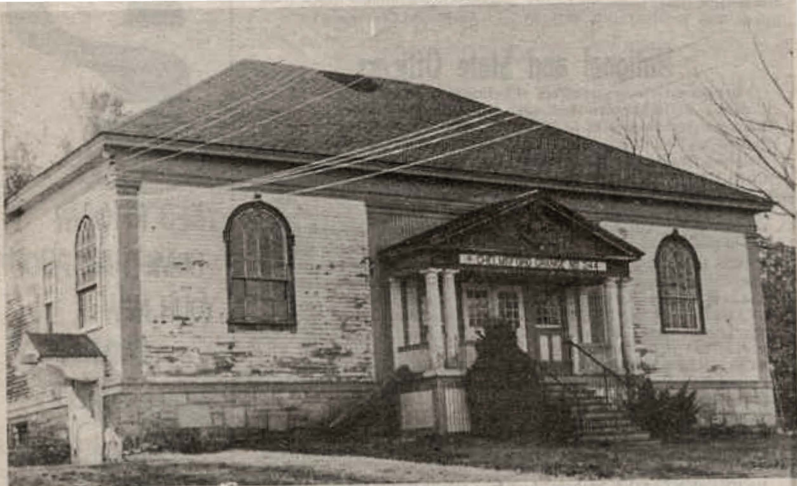
THE OLD GRANGE HALL on Proctor Road will have as its principal tenant from now on, the Girl Scouts. The Selectmen made the decision Monday night, Nov. 15. A good deal of renovation work will be done (most of it waiting until Spring) and a number of restrictions were placed upon use of the property. Scout leaders at the meeting were very pleased with the decision. (Photo by Rob Macentee)
