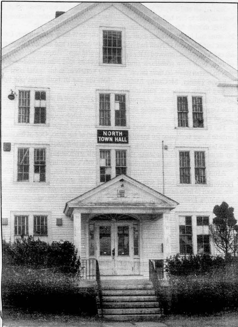
FORGOTTEN PAST: The old North Town Hall seems to have been forgotten. It sits across from the North Chelmsford Fire Station needing a coat of paint, new windows and other repairs. (Photo by Sue Ellen Woodcock)
